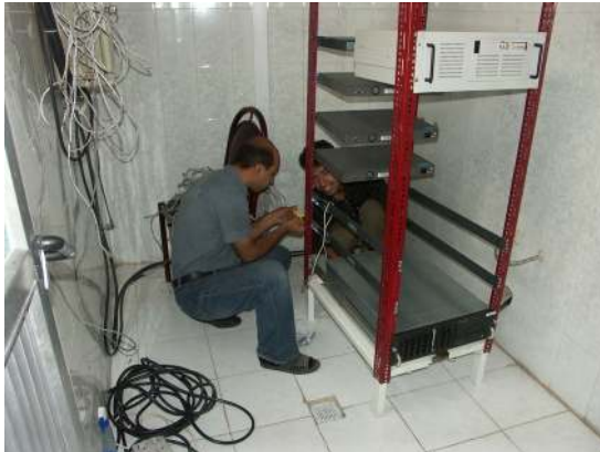
Server room at Computer Science Faculty, Herat, 2005
